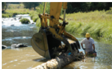
Highland Trucking Co. employee, Anthony Lambert, helps direct log placement for aquatic restoration work at The Nature Conservancy's preserve on the Middle Fork John Day River. Photo © The Nature Conservancy/Jim Yuskavitch
