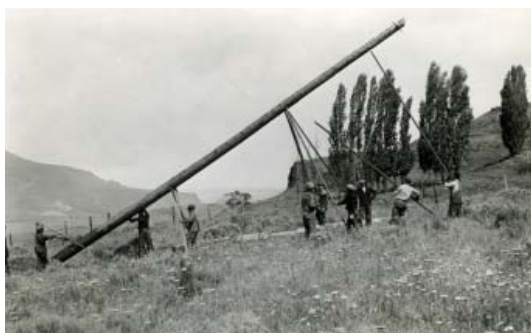
Getting electricity to rural customers was part of Pacific Power's early rural electrification program.
