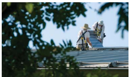
Blue Sky supported installing a 40-kilowatt solar array at Walla Walla's Whitman College in 2009.
