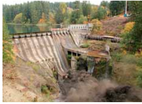
Stored water gushes through the tunnel created in the Condit Dam in Washington.
