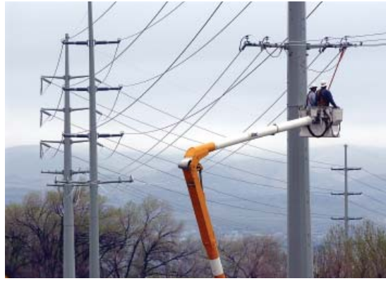
Pacific Power makes wise investments in the electric system in order to deliver safe and reliable electricity today and into the future.
