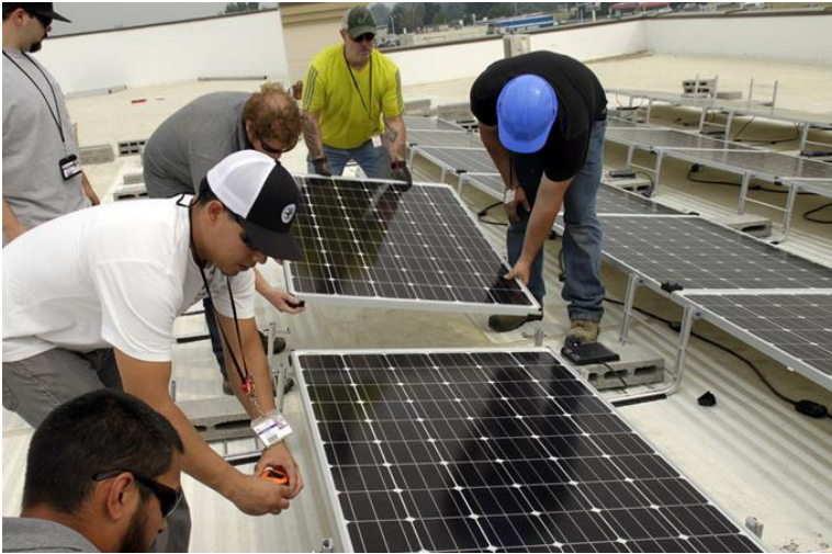
Perry Technical Institute, 15.68 kW solar array
