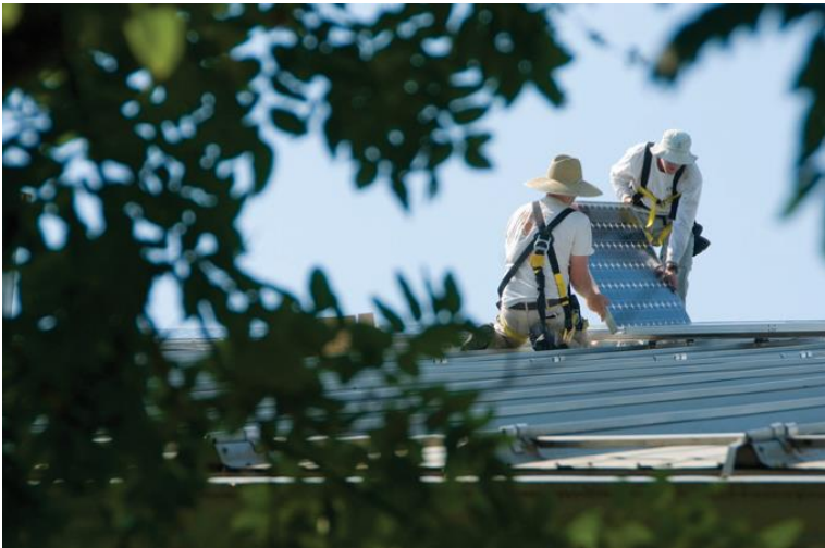
Whitman College, 21 kW solar project
